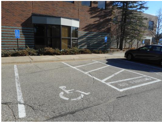
Photo 1: Accessible parking spaces have been designated near the main entry. This is a good example of accessibility. Currently 2 of the spaces are missing signs designating the accessible parking and 3 of the signs are not centered on the parking space.
