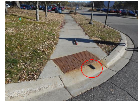
Photo 3: Curb ramps are provided in order to create an exterior pedestrian route from Williston Rd. to the main entry. The existing curb ramps are in rough condition and have up to 30% slope along the gutter at some locations.
