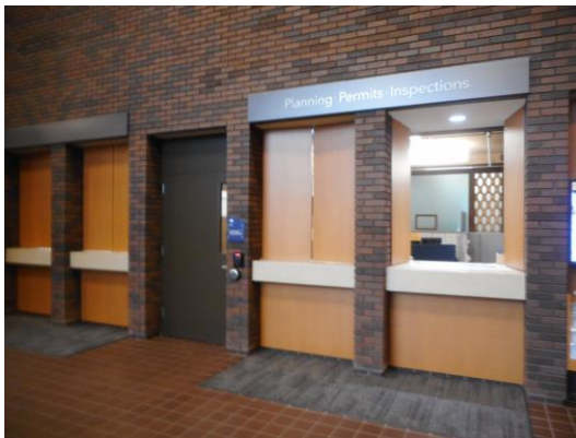
Photo 4: Service counters for City Clerk, Planning / Permits / Inspections and Utility Billing & Assessing are currently at 42" AFF (vs. 36" maximum).
