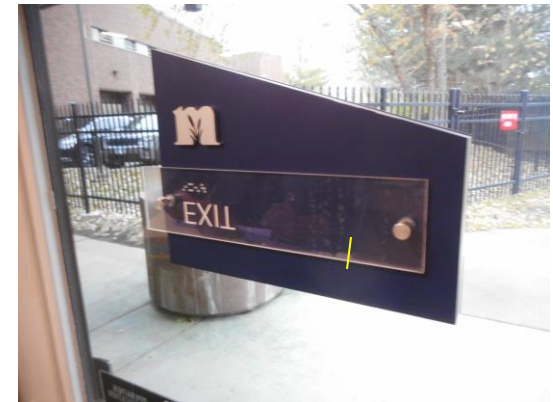
Photo 12: The sign stating "Exit" from within the break room is installed backwards, with the tactile and braille characters facing the in to the wall (as well as the "T" being upside down).
