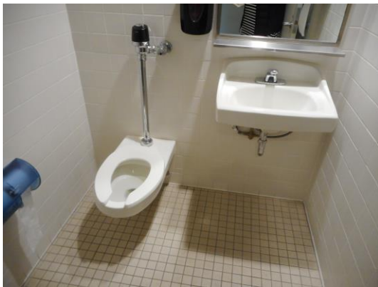
Photo 16: There are additional single-user toilet rooms located near the Mayor's office and in the kitchen area. These single-user toilet rooms currently provide no features of accessibility and are too small to provide compliant clearances at fixtures.
