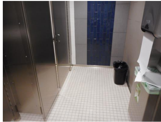
Photo 8: In the lower-level women's toilet room the towel dispenser/waste receptacle unit reduces the width of the maneuvering clearance on the pull side of the accessible compartment door.
