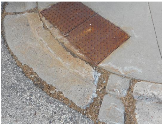
Photo 4: The rough condition of the curb ramps includes crumbling concrete and an abrupt transition where the concrete gutter meets the asphalt drive lane.
