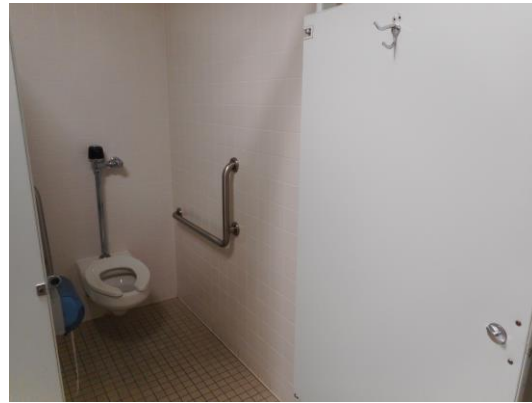
Photo 14: The multi-fixture toilet rooms currently provide minimal features of ambulatory accessibility. Providing a wheelchair accessible compartment in these rooms would require the elimination of fixtures, which may not be possible due to other code requirements.
