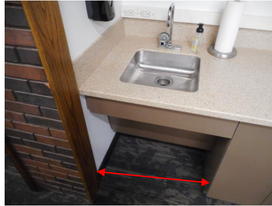
Photo 14: At the coffee station with the Community Development department a sink with a forward approach is provided (a parallel approach is not possible due to the adjacent wall). This is a good example of accessibility. The width of the clear floor space is only 29" (vs. 30" minimum) due to the trim detail on the brick wall.
