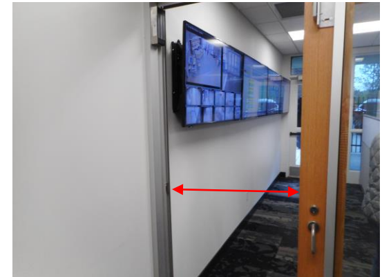
Photo 9: The sliding door to the IT and security office provides a 31" clear opening (vs. 32" minimum) due to the electronic door lock mounted on the top. The TV monitors within the space protrude 6" into the circulation route (vs. 4" maximum).
