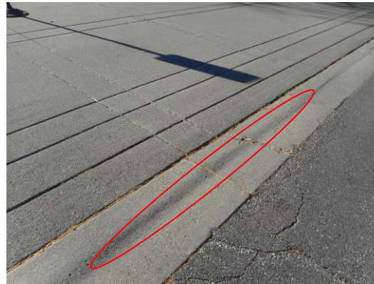
Photo 2: A flush curb is provided along the full width of the sidewalk leading to the entry. This is a good example of accessibility. Currently there is an abrupt rise and short (~3") steep section along the gutter (>21% vs. 8.33% maximum).
