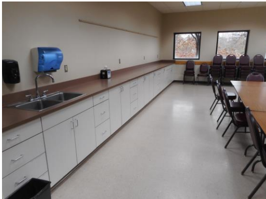
Photo 10: The sink in the Minnetonka Mills room is currently at 36 1/4" (vs. 34" maximum) and does not allow for a forward approach with knee and toe clearance.
