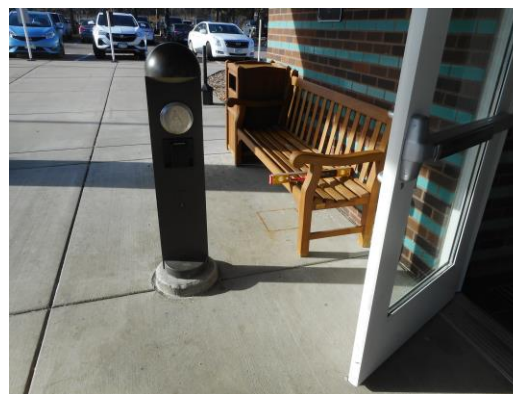
Photo 5: A power door operator is provided at the main entry. This is a good example of accessibility. The arc of the door swing currently overlaps the clear ground space for the control button and the control button is currently mounted approximately 4" too high (it is mounted on a concrete base, different than City Hall).
