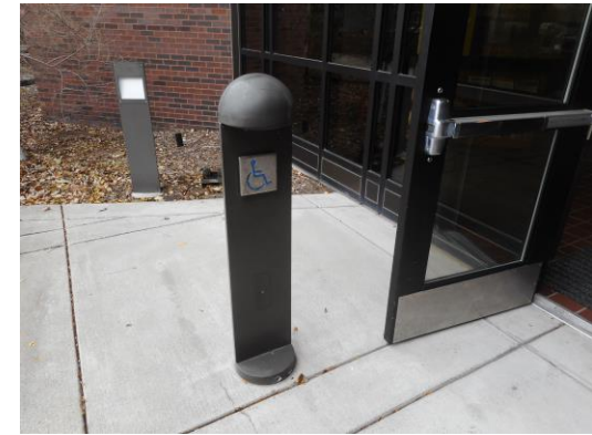
Photo 3: A power door opener is provided at the main entry. This is a good example of accessibility. Currently the arc of the door swing overlaps the clear ground space at the control button.
